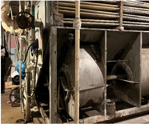
HVAC equipment requiring replacement
