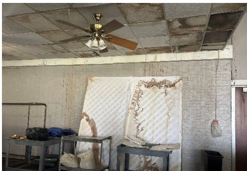
Water damage from leaking roof
