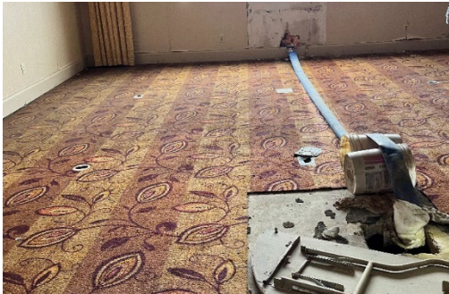
Conference center sinkhole
