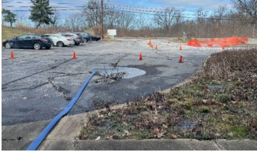
Front parking lot sinkhole
